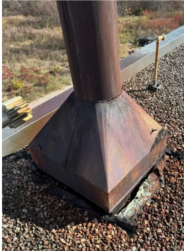
Figure 7 – Roof Vent Stack Close Up
